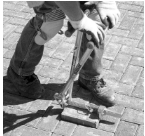
Figure 10. During initial compaction, cracked pavers are removed and immediately replaced with whole units.
