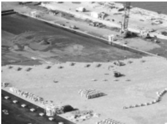
Figure 7. Maintaining an angular laying face that resembles a saw-tooth pattern facilitates installation of paver clusters.
