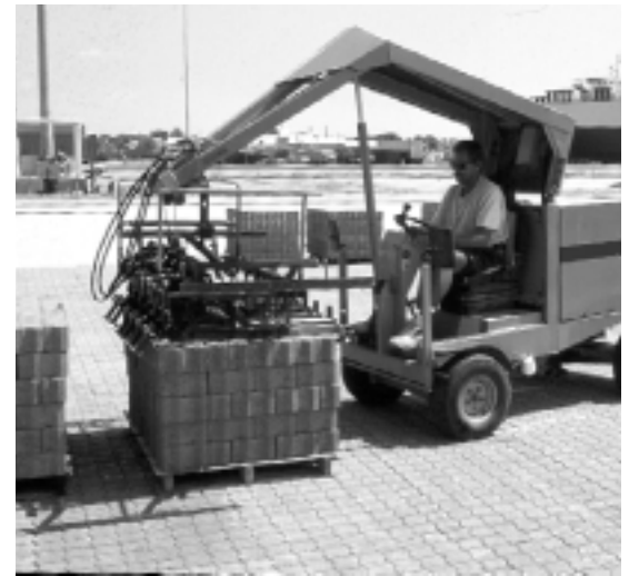
Figure 3. A cluster of pavers (or layer) is grabbed for placement by mechanical installation equipment. The pavers within the cluster are arranged in the final laying pattern as shown under the equipment.
